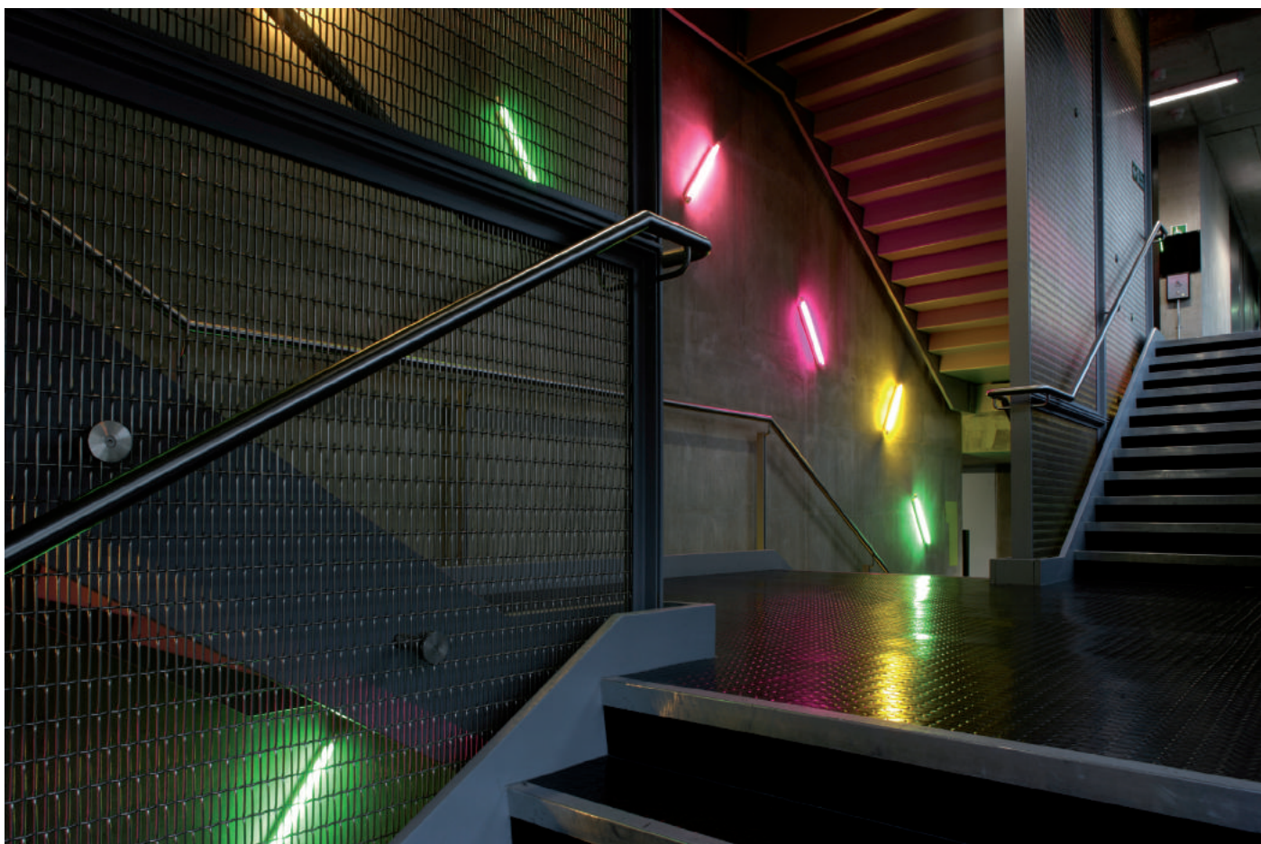
Scissor stair lighting
